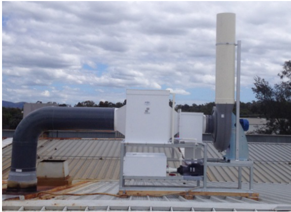
Roof mounted Advanced Air® fume scrubber 1200L/s.
