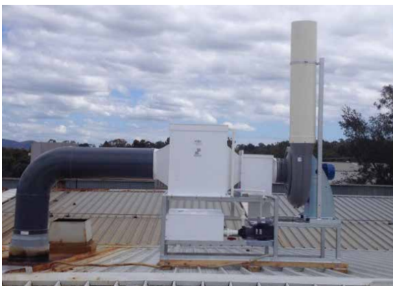
Roof mounted Advanced Air® fume scrubber 1200L/s.
