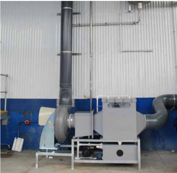
Advanced Air® fume scrubber 900L/s.
